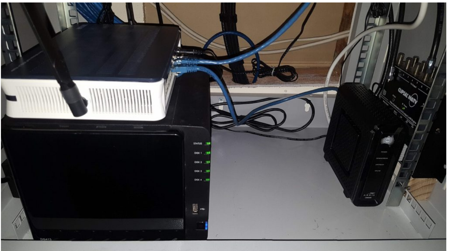
Photo 5: Bottom of cabinet with the old power boards removed, thereby freeing up some space. You can see the Synology NAS on the left with the Billion Router on top and the Arris NBN modem to the right.
