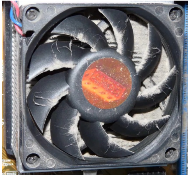
Figure 14 – Dust accumulated on the fans leading edge.
